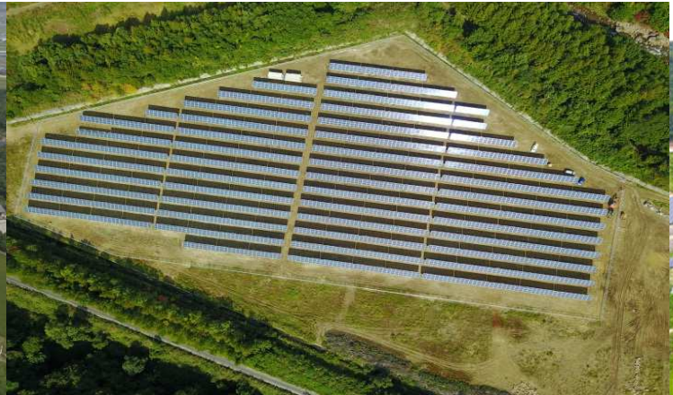
Fukushima Inawashiro solar power plant 1.2MW
