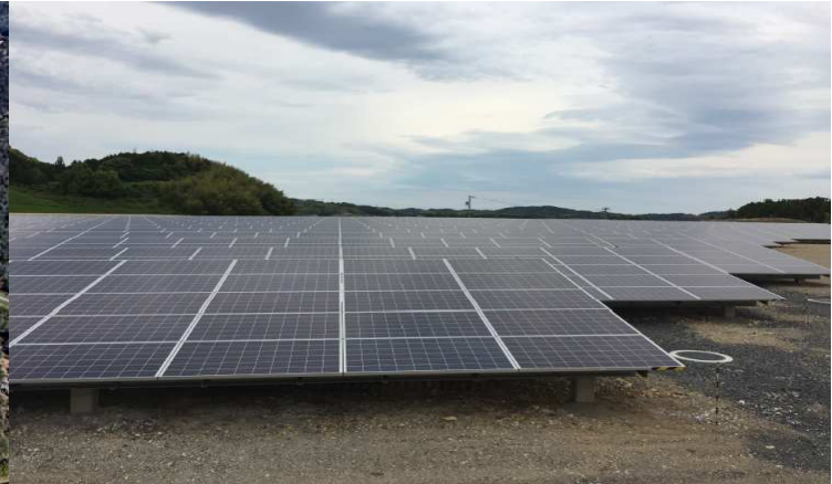
Mie Taki-cho Nonaka solar power plant 1.2MW
